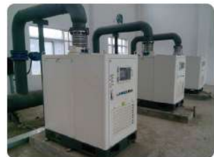
Sewage treatment plant in Gaoyou
